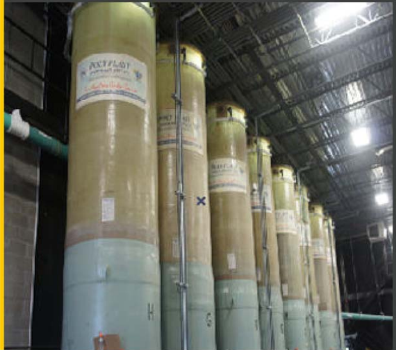
Ion Exchange Column 1.8 m dia x 5.4 m height - 16 nos.
